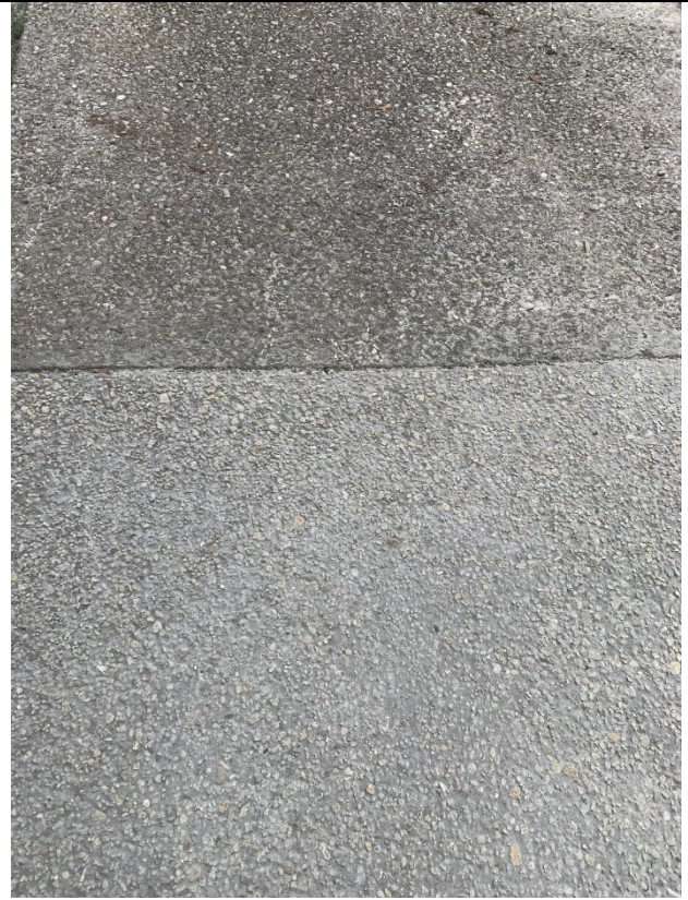
Concrete install (matching new texture to existing. (Existing path is on top and the new is below) We are happy with how well they match.
